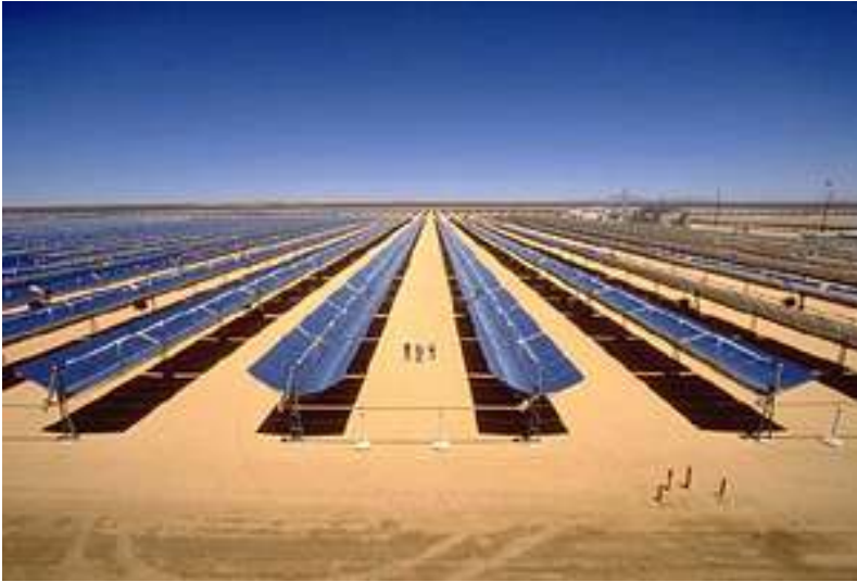
Engineers working at the Solar Energy Generating Systems (SEGS) facility in the Mojave Desert
